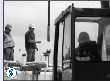
Following hand signals from Chugach rigger/director, Brad Trumbull, Everet Seeley at controls of crane, removing inoperative pump from above ground fuel tank.
